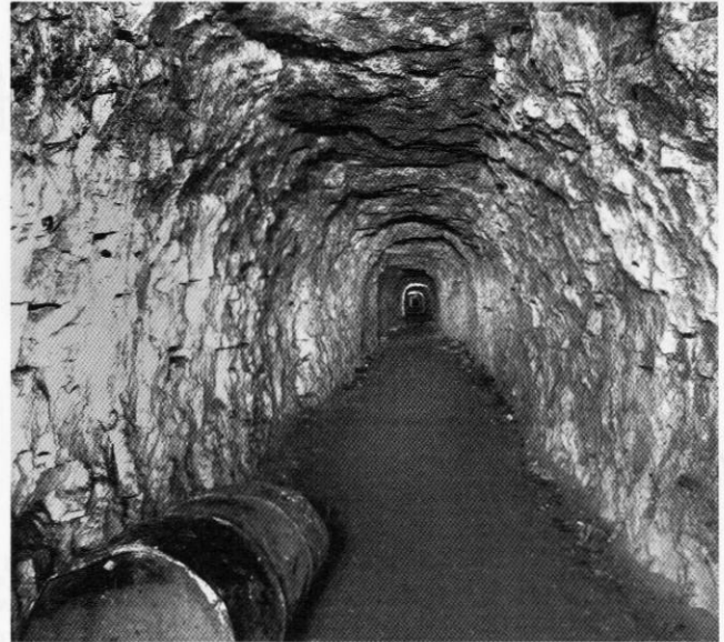
Looking west along the first section of new shelter tunnel. The standard-gauge railway tunnel is behind the photographer
